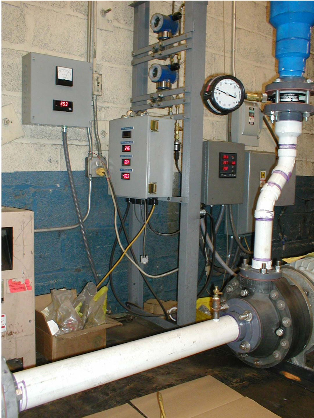
Figure 1. Pump on the Test Stand.
